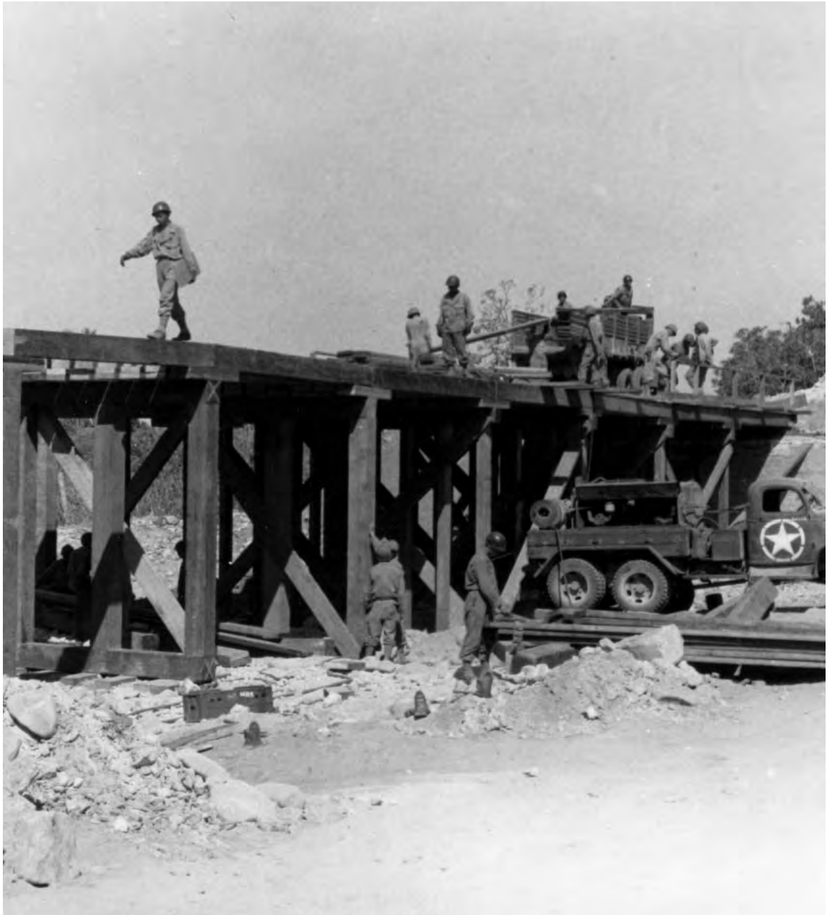
BRIDGE BUILDING. In the valleys this task presented no particular problem once the enemy had been chased off the mountain ridge overlooking the bridge site. However, near Messina, where the road in some places is hewn out of the cliffs overhanging the sea, the problem was more difficult. The air compressor (Le Roi) mounted on a 2 \frac{1}{2} -ton truck (in picture above) was used for operating power-driven saws, hammers, and drills.
