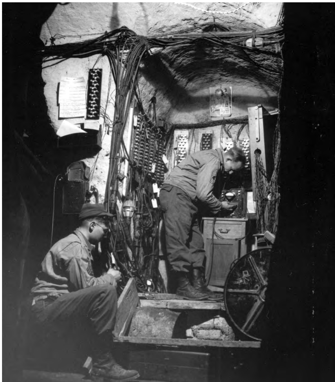
SIGNAL CORPS MEN working in the main frame room of headquarters switchboard installation. The beach area at Anzio-Nettuno was on a slightly higher level than the rest of the beachhead area and was honeycombed with tunnels and caves so far underground that they were bombproof. Wherever possible the installations along the shore were put underground.
