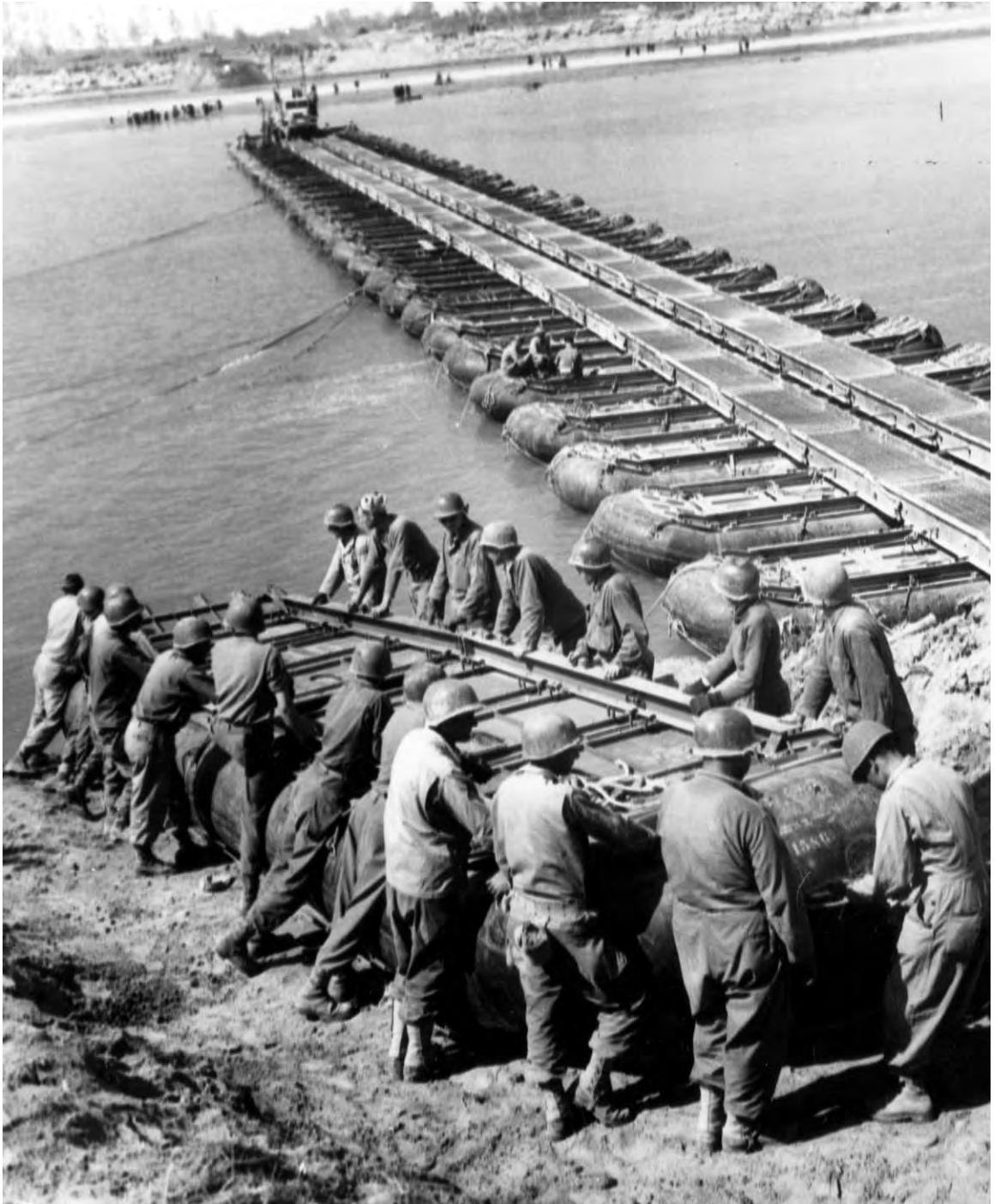
PONTON BRIDGE under construction across the Po River near Ostiglia. This bridge was opened on 25 April. (M2 treadway bridge.)
