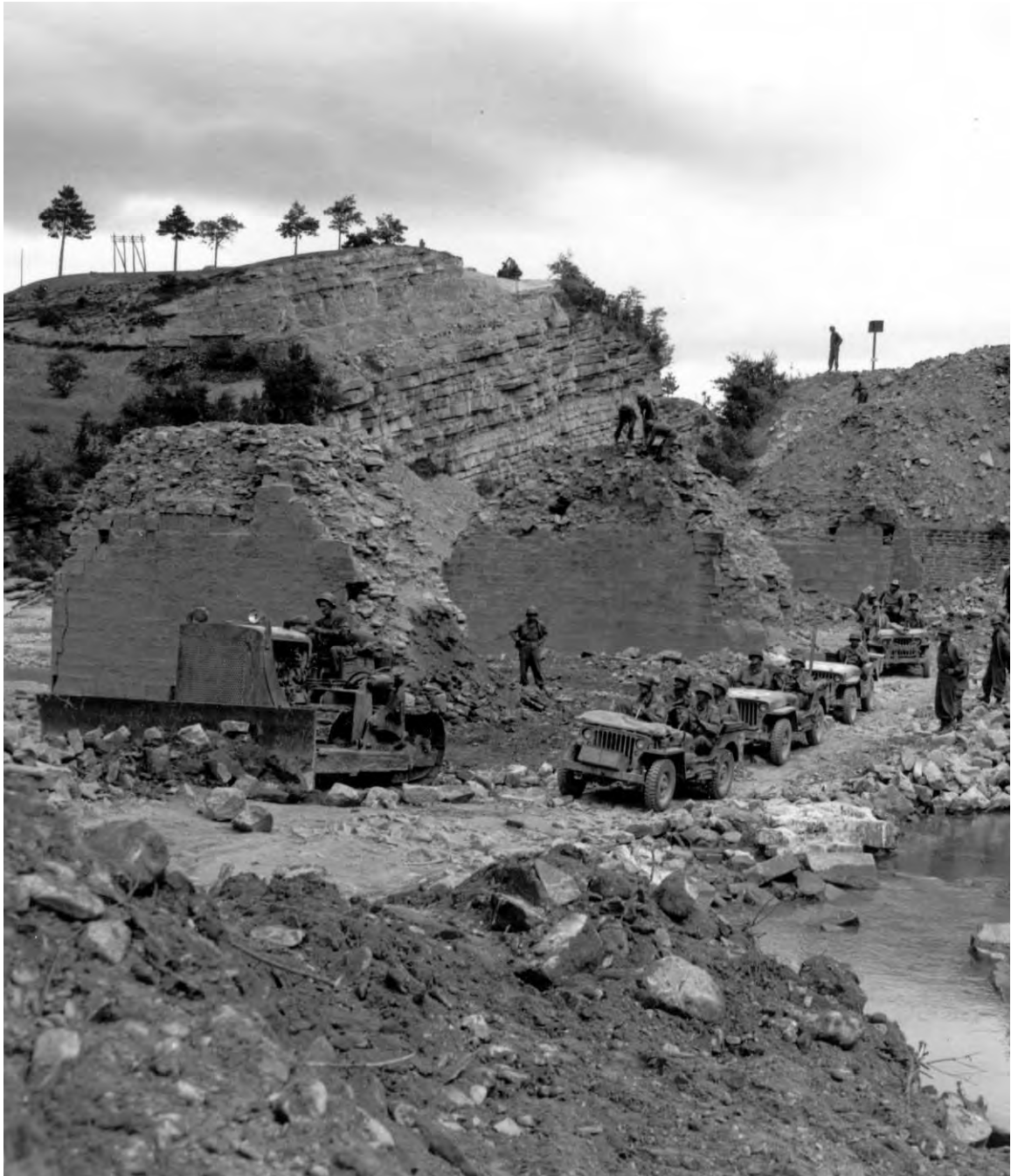
AMERICAN ENGINEERS CONSTRUCTING A BYPASS in the Firenzuola area during the pursuit of the Germans. The combat engineers, prepared to bulldoze a bypass or to install temporary bridges, followed closely behind the leading elements of the infantry and armor. (Jeep; crawler type diesel tractor with angledozer.)
